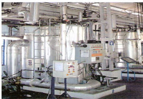
Thermic Fluid Heater
