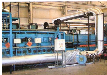
Waste Heat Recovery System In Decarb Furnace
